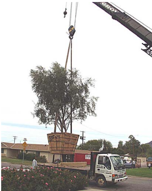
Lower the tree into the planting hole using equipment and manpower appropriate to the task.
