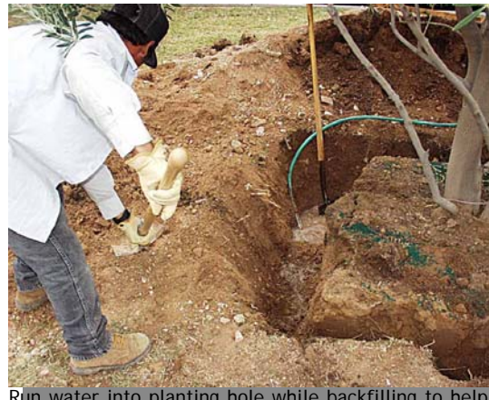
Run water into planting hole while backfilling to help settle the backfill and avoid voids or air pockets. Tamp frequently.
