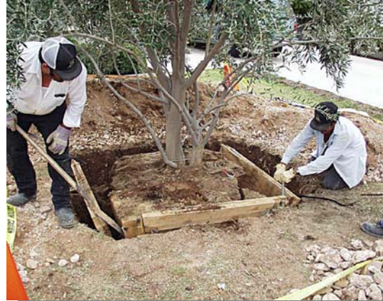
Backfill around box about half way up and tamp soil. Then remove box sides.
